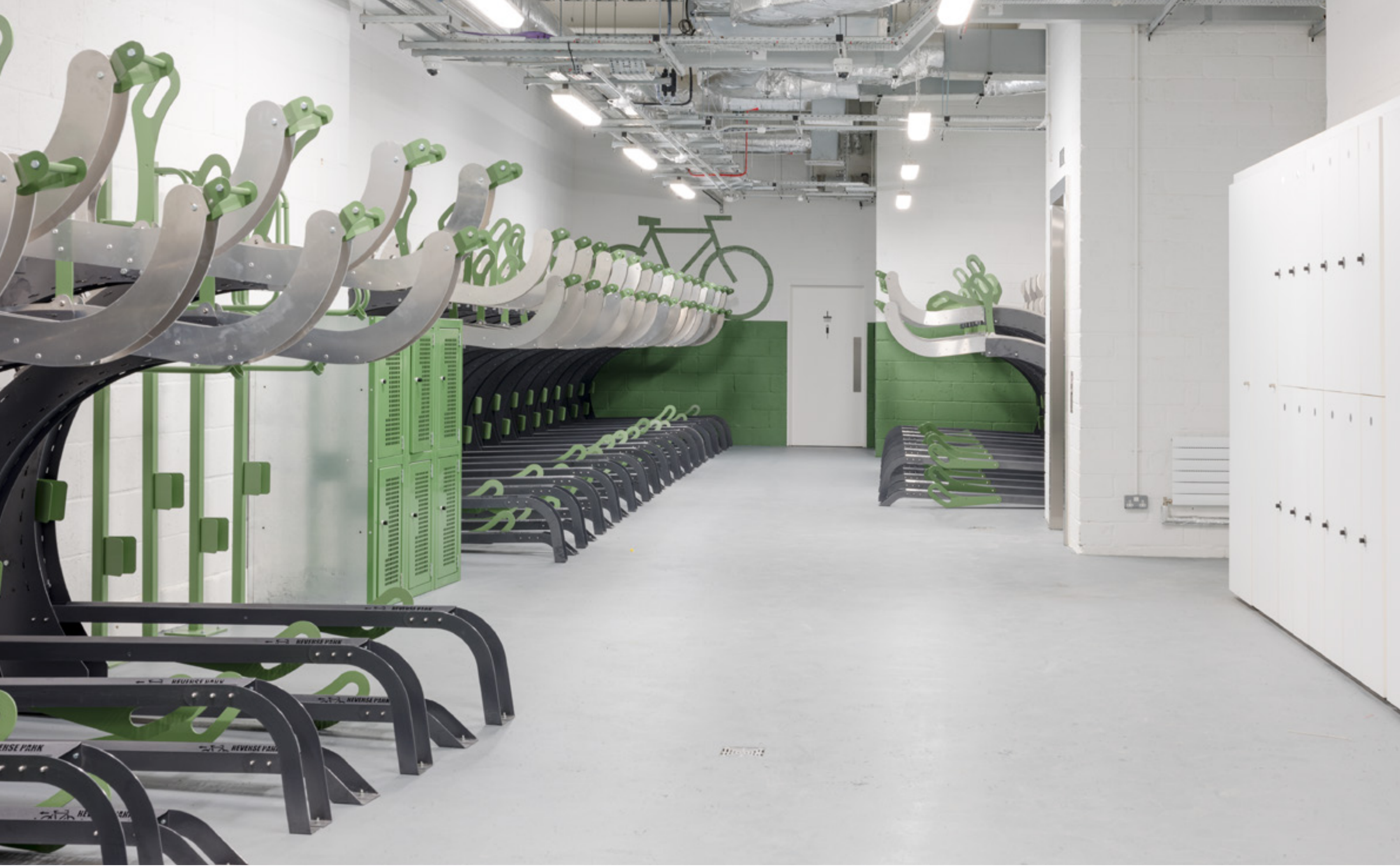
146 ARC CYCLE RACKS BY FIVEATHEART, AT 459 SQ FT OF NET OFFICE SPACE PER RACK
